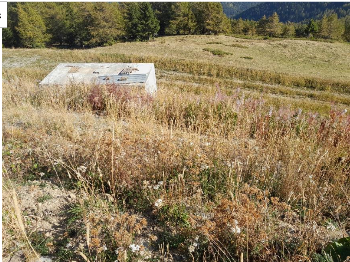
POINT DE RACCORDEMENT – ALIMENTATION ELECTRIQUE
