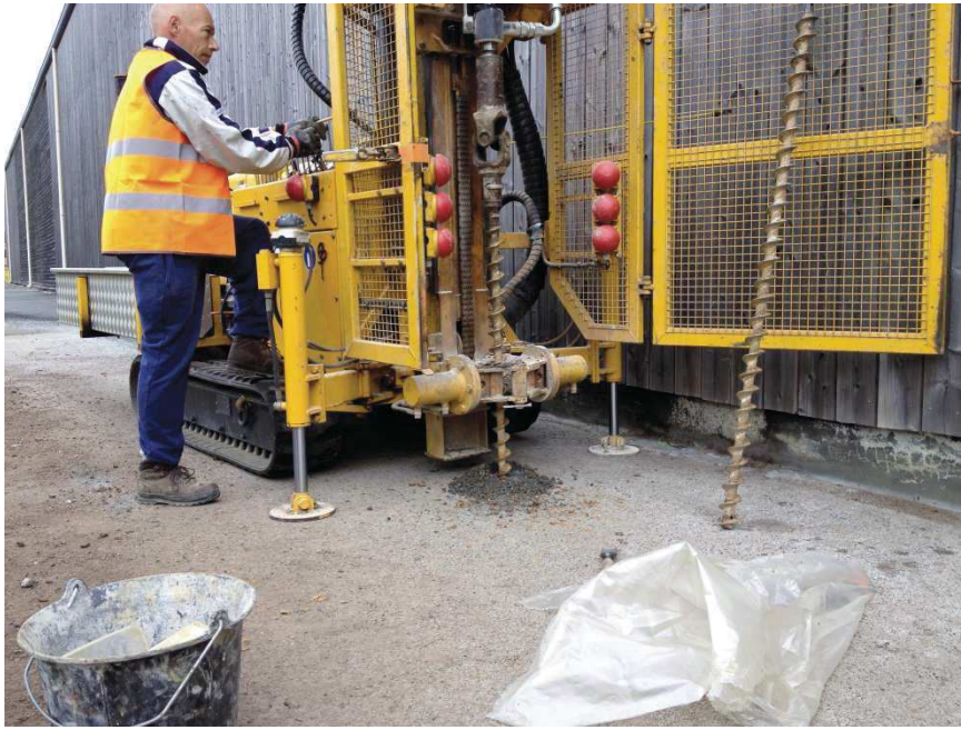
Photo 5. BH4 location at the back of the autoclave building and on a stain on the asphalt
