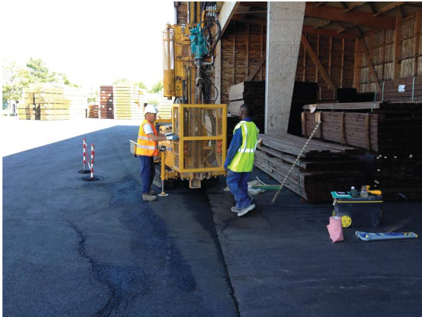
Photo 4. BH3 location at a stain on the asphalt
