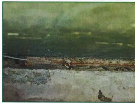
Figure 45 : AA-P4-RG - Corrosion des frettes
