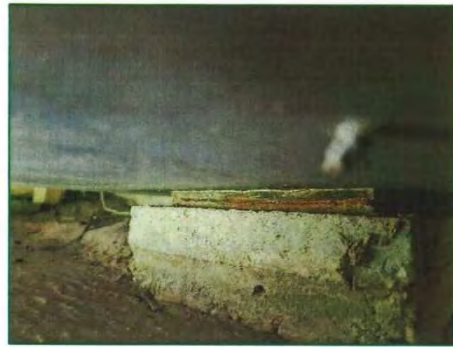
Figure 43 : AA-P3-RD - Corrosion des frettes
