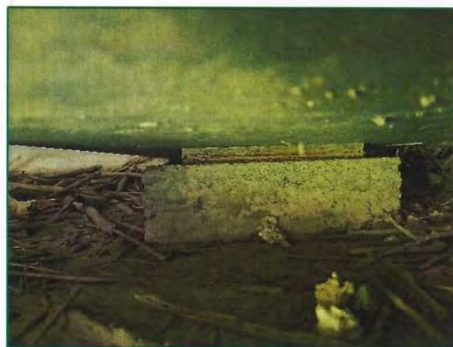
Figure 47 : AA-P2-RG - Corrosion des frettes
