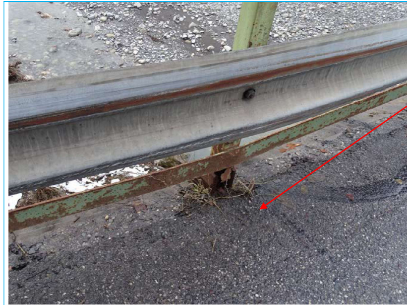
Photo 19 Extrados amont RD Eraflures Tassement
