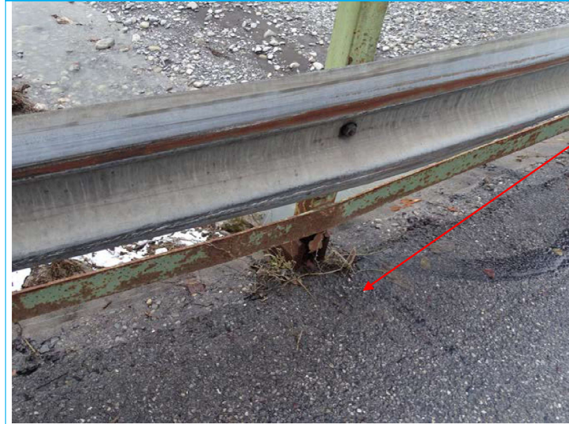
Photo 19 Extrados amont RD Eraflures Tassement
