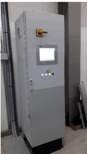
Picture of the A2.400 Control panel:
