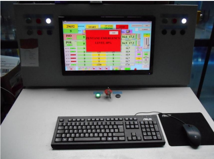
Picture of the 40% level detection emergency screen available from the main computer supervisor. Because of power off in the computer due-to the emergency situation, the message will be available only after the normal and safe condition will be re-established.
