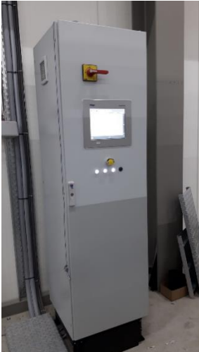
Picture of the DRAGER detection system in front of the A2.40 control panel
