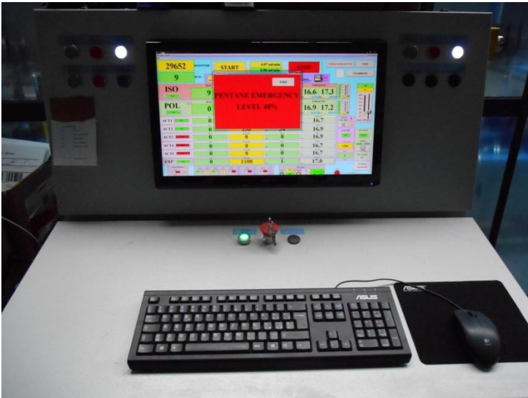
Picture of the 40% detection level available from the main computer supervisor in case of emergency detection on the Pentane storage section
