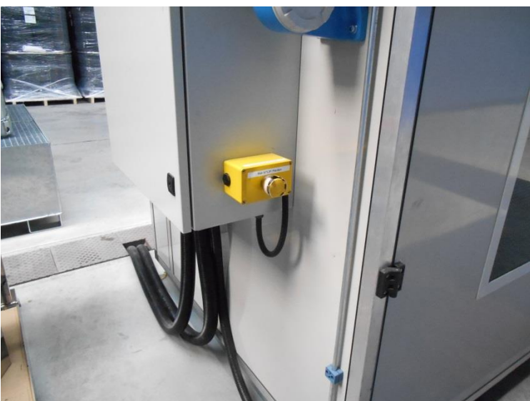
Picture of the yellow Pentane emergency button located on side of the Pentane pump cabin.
