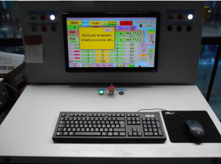
Picture of the 20% detection level screen available from the main computer supervisor in case of warning detection on the Pentane storage section
